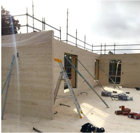
Assembly of external wall panels (IsoTimber + CLT) with floor panels (CLT) © Gustab AB
